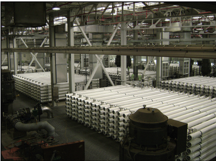
Reverse osmosis vessels take the microfiltration effluent and turn it into pure water that will be pumped out to spreading grounds and returned naturally to the drinking water supply.
